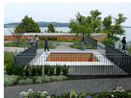
Custom-made guardrails were installed on the ZinCo Guardrail Bases all along the atriums and any other edges.
